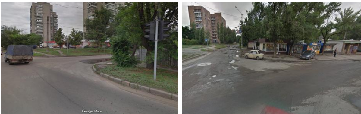
Fig. 3. Current condition of the road surface on Silikatna St. (Kharkiv)
